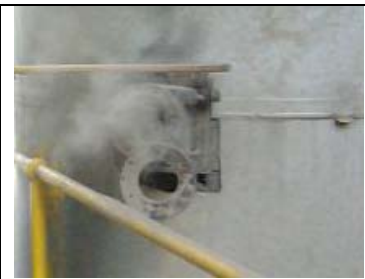
Photo 2: Backing of ash in the next loop seal.
